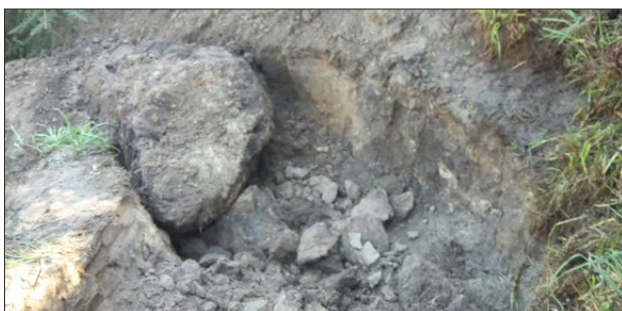
One of the boulders blocking the track
